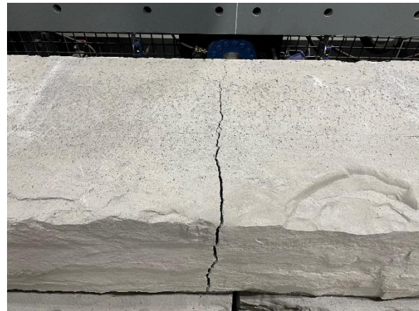
Figure 6 – 6 ft block cracked under high load
