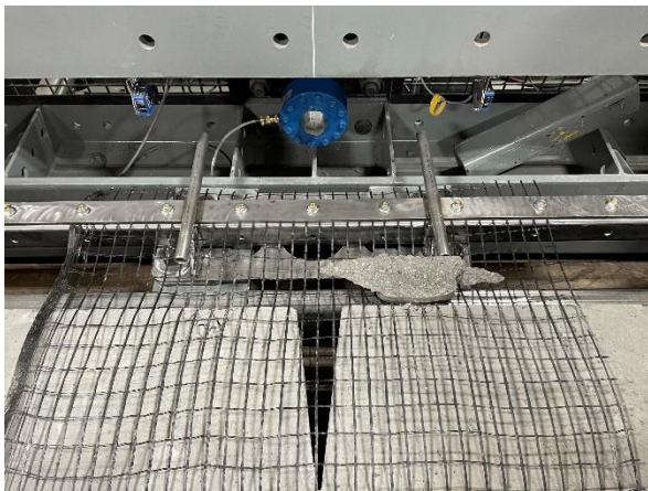
Figure 4 - Shear heel sheared off
