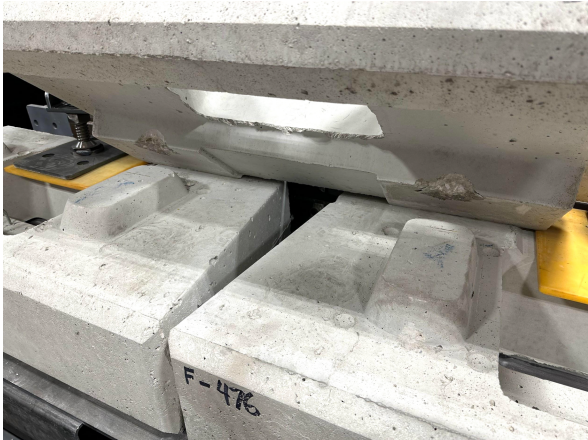
Figure 3 – Groove crushing at shear knobs
